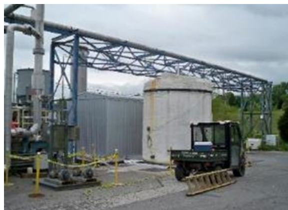
Figure 3.16. The Chromium Water Treatment System
