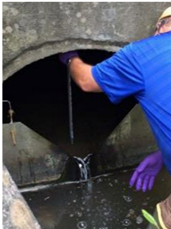
Figure 3.13. Storm water outfall monitoring
