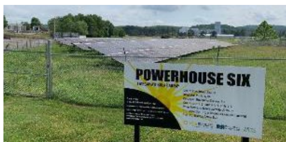
Figure 3.5. Oak Ridge Powerhouse Six Solar Farm
