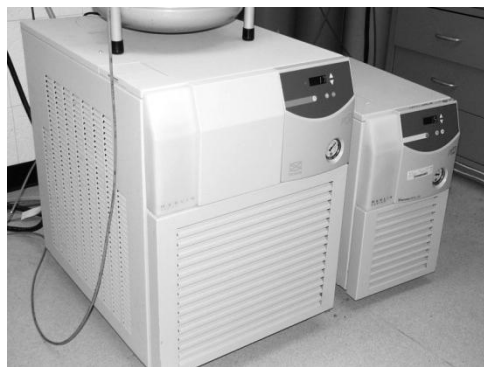
Fig 5.5. New closed-loop chilled water systems.
