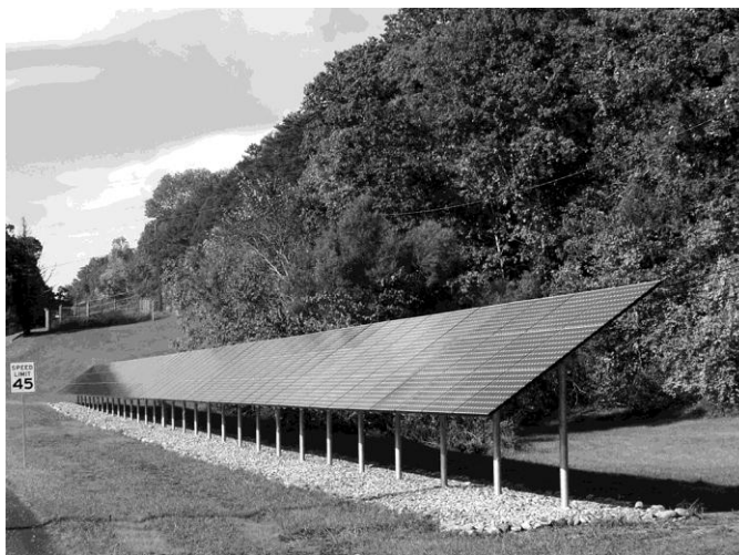
Fig. 5.4. The solar array installed in 2008 at ORNL generates 51.25 kW at peak power.
