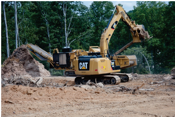
Fig. 4.14. Uranium Processing Facility site readiness construction is using a mulcher/chipper to produce mulch that is being used as erosion control along the haul road.
