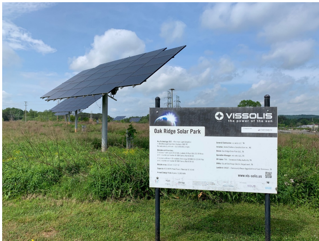
Figure 3.5. Oak Ridge Solar Park
