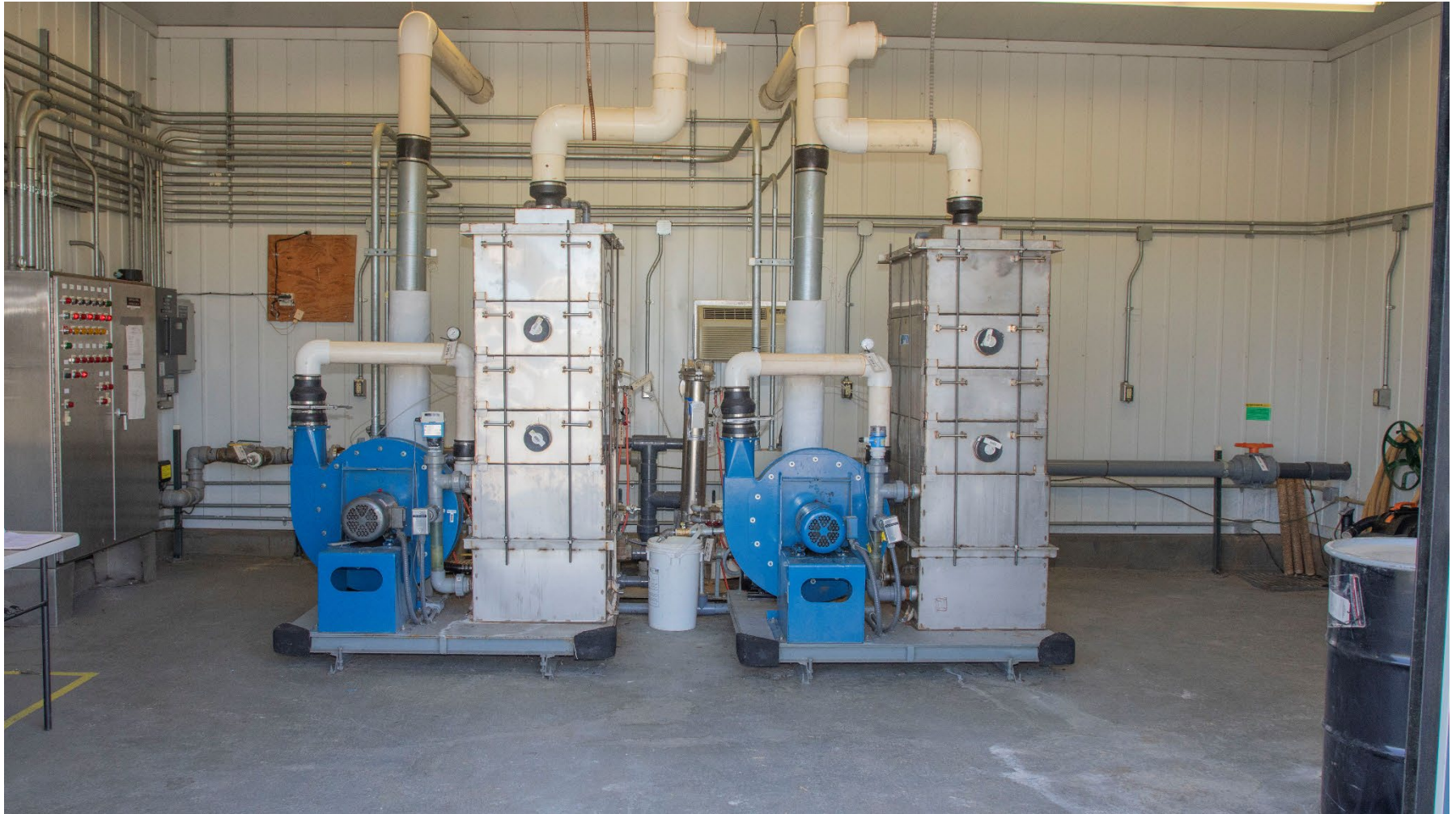
Figure 1. Inside the EEVOC treatment facility building.
