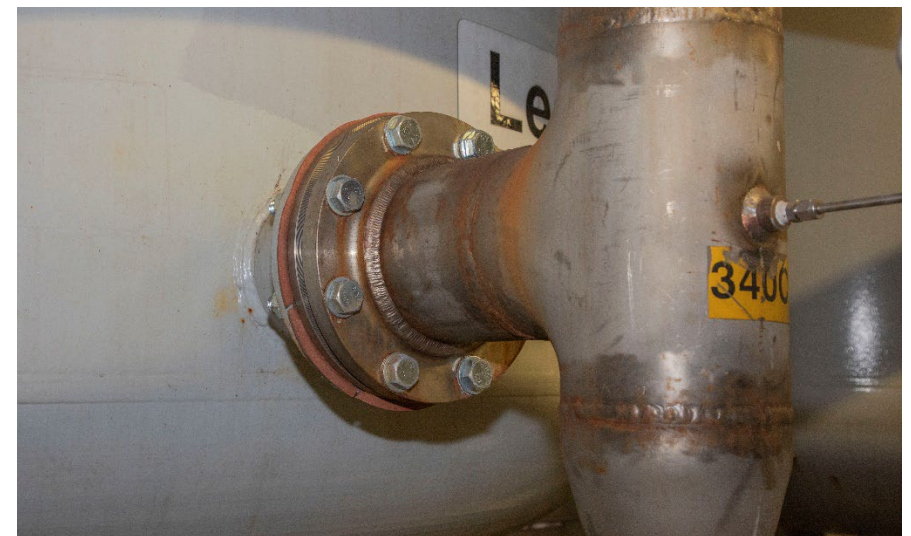
Figure 4. Close-up of flange with zinc-coated carbon steel replacement bolts.
