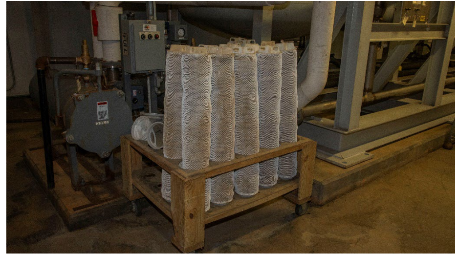
Figure 2. Spent pre-filter cartridges drying prior to disposal.
