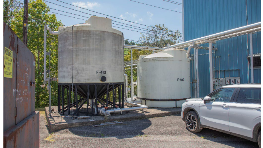
Figure 6. BSWTS backwash hold tank (F-410) and backwash feed tank (F-400).
