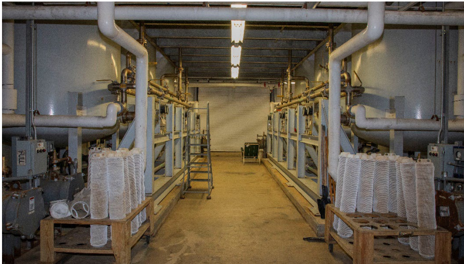
Figure 3. View of treatment system left and right bank carbon columns.
