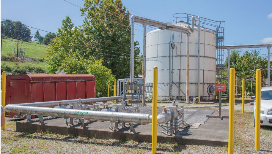
Figure 5. Wet well (foreground) and equalization tank outside of Building 9201-2.
