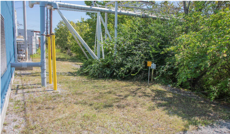
Figure 7. BSWTS discharge to UEFPC.
