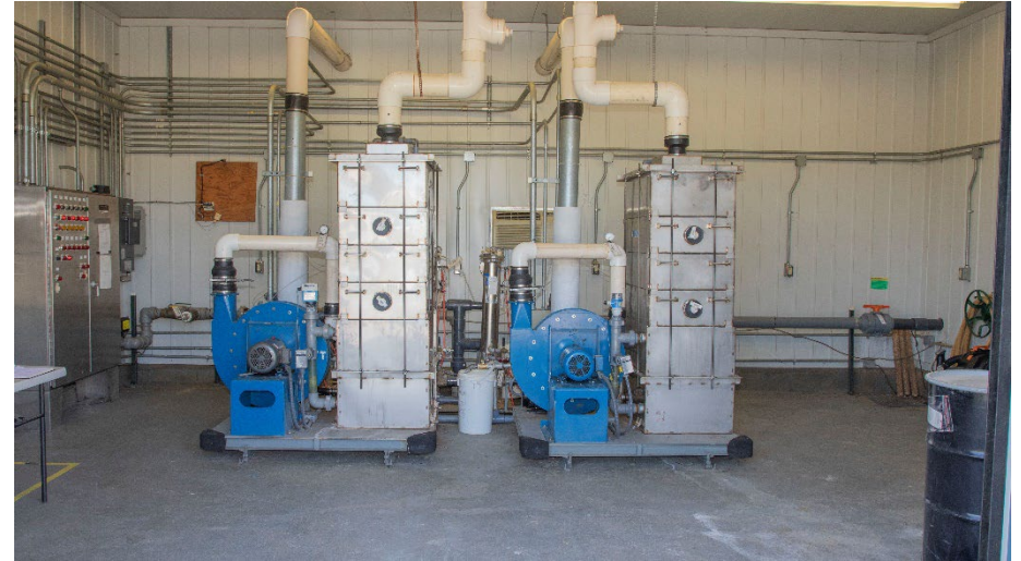
Figure 2. EEVOC air strippers inside the treatment facility building.
