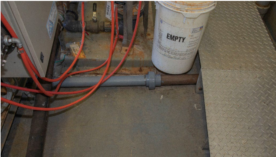
Figure 3. Discharge pipe showing clear plastic section to monitor scale buildup (below bucket in photo) inside the treatment facility building.
