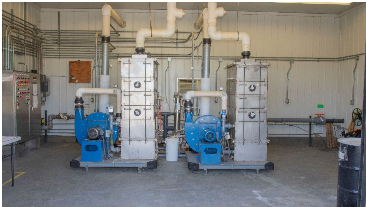
Interior view of treatment system building
