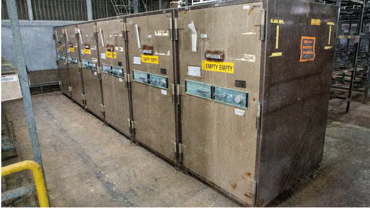
Figure 6. Storage safes (YPH-24-1150974)
