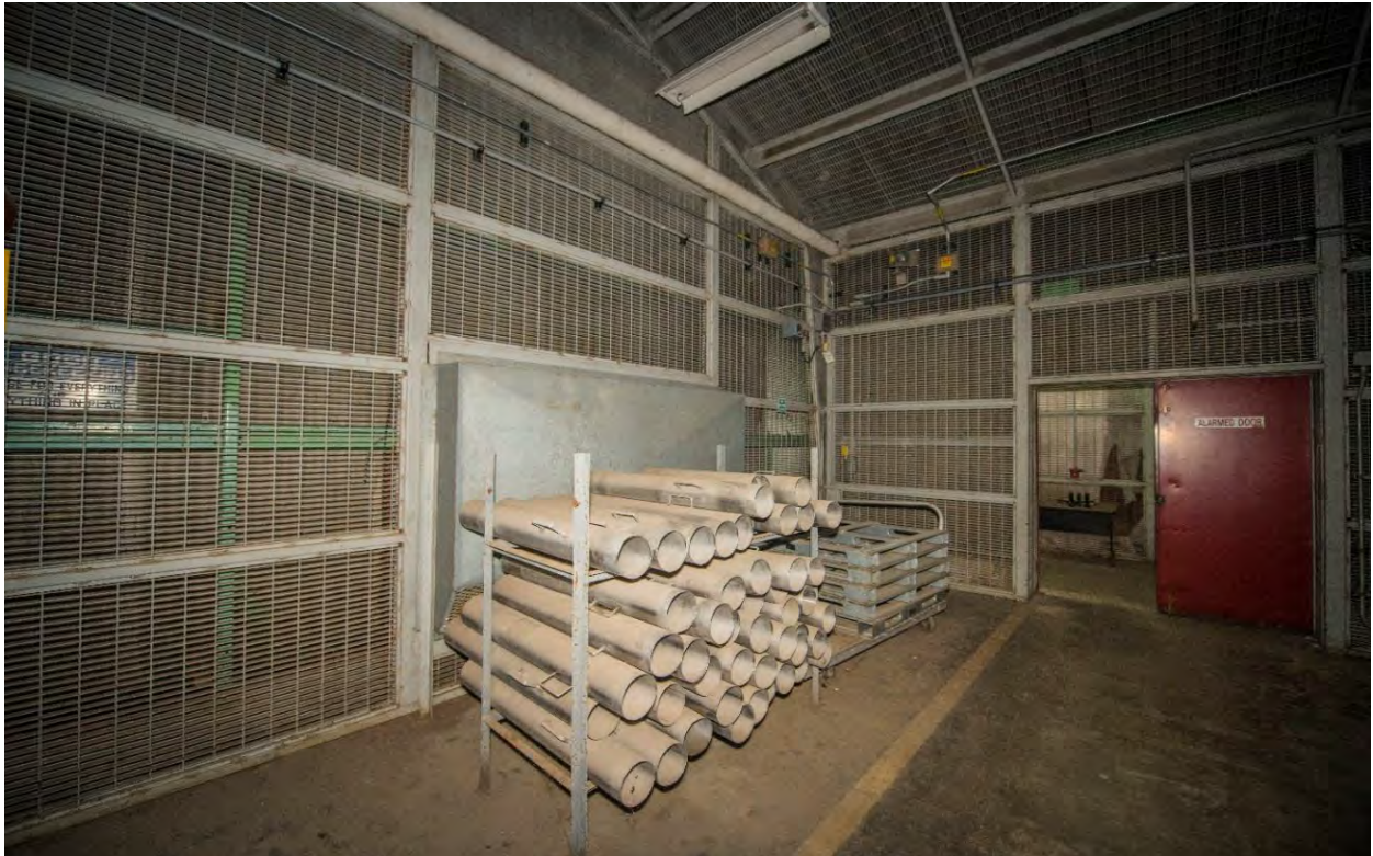
Figure 7. Safe bottle carriers and storage rack, pallets, and pallet cart (YPH-18-810989)
